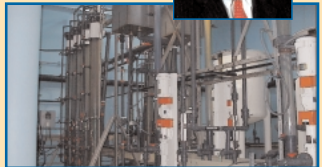
Houston's dual train 22-gallon-per-minute pilot plant allows the evaluation of new treatment technologies.
