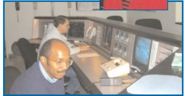
Norfolk Utilities Waterworks Operators monitor the water treatment process using a Supervisory Control and Data Acquisition (SCADA) system.
