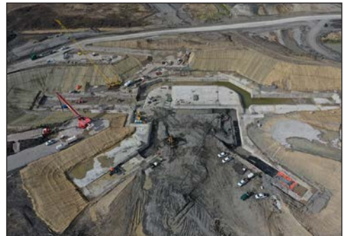
TOP: 72-inch Water Transmission Parallel Pipeline
