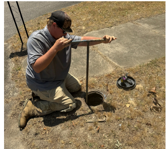
TOP: A utility worker performs a lead service investigation in compliance with EPA's Lead and Copper Rule Revision.
