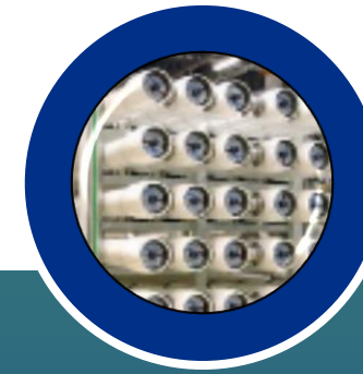
Reverse Osmosis Membranes
