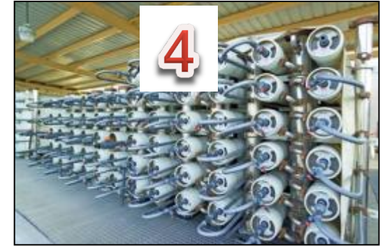
RO (Single): Refinery
