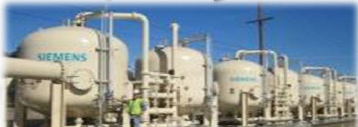
SF Groundwater Basin Remediation
