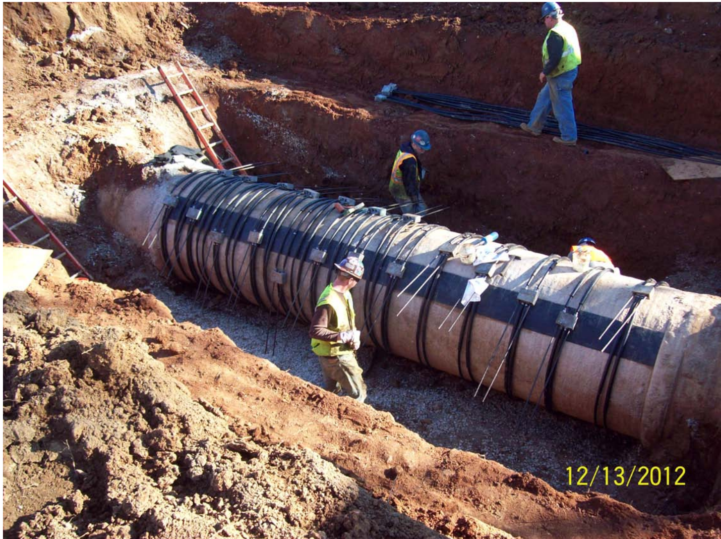
external post tension,
