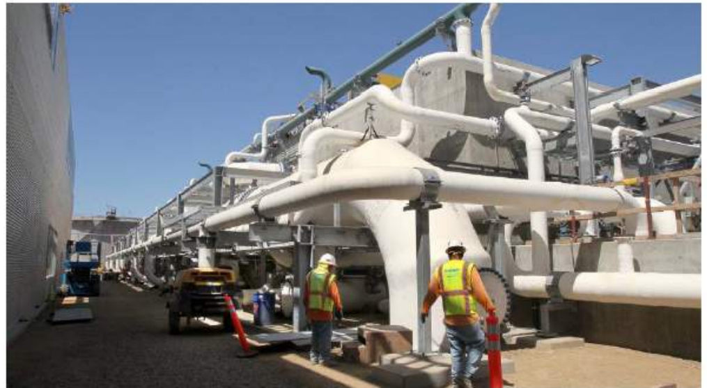
View of some of the hardware at the Carlsbad Desalination Project. — Charlie Neuman
